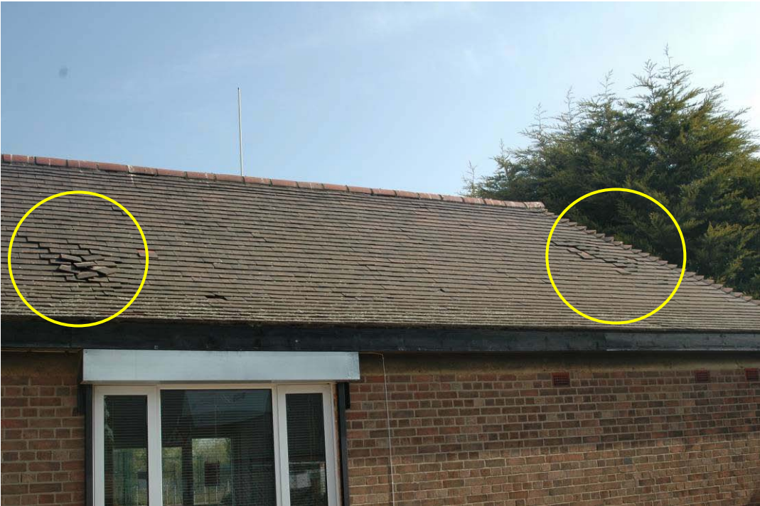
Figure 4.3: Areas of Damage
