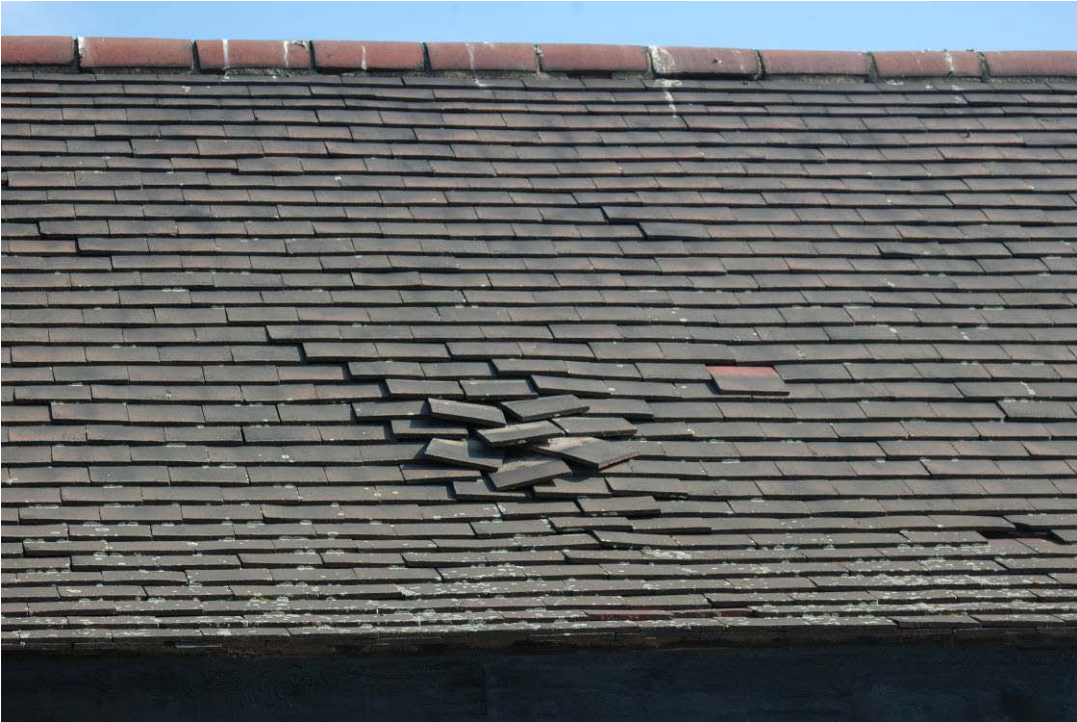
Figure 4.2: Main Area of Damage to Roof of Marina Building
